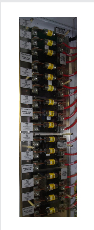
SGI 500 with 16 fused positions, 4 - 150A fuses, 4 - 125A fuses, and 8 - 175A fuses
