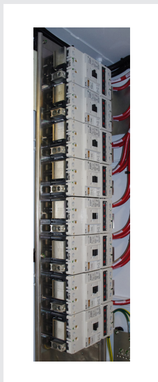
SGI 500 with 8 breaker positions, 7 - 400A breakers, and 1 - 350A breakers
