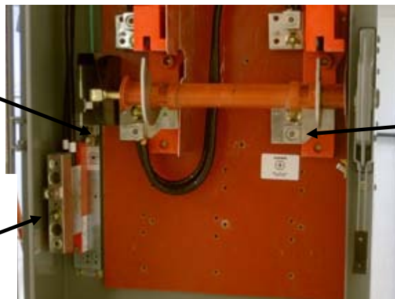
Fig. 6 DC disconnect without a Fused PV Sub-combiner option.
