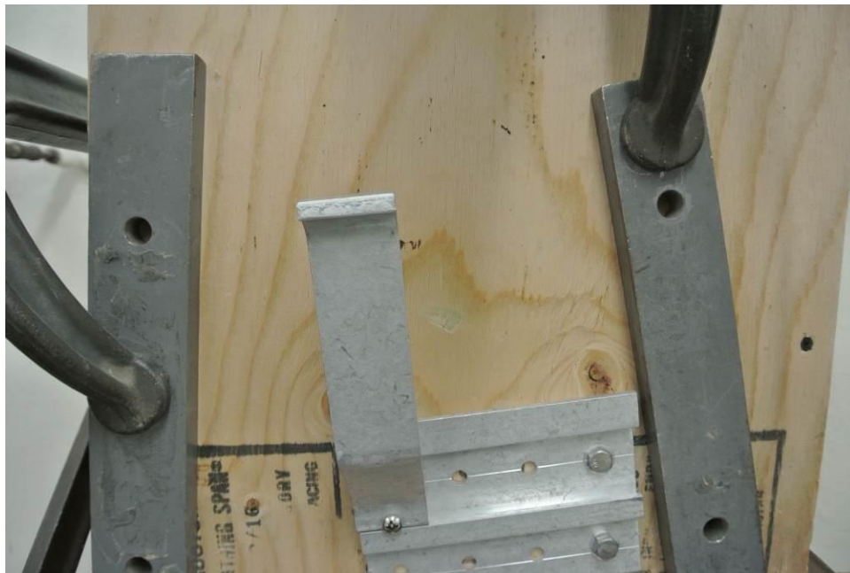
Figure 3b. Typical Failure Mode
